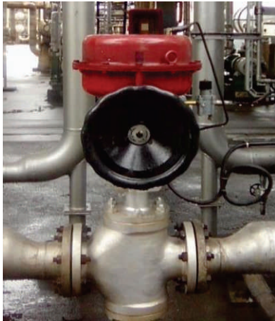
Figure 4: Pneumatic Crude Control Valve.
